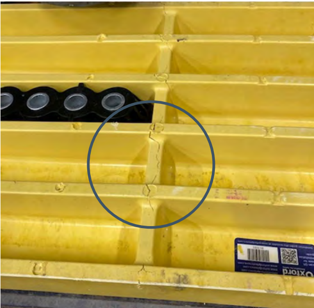
Crack along rib
