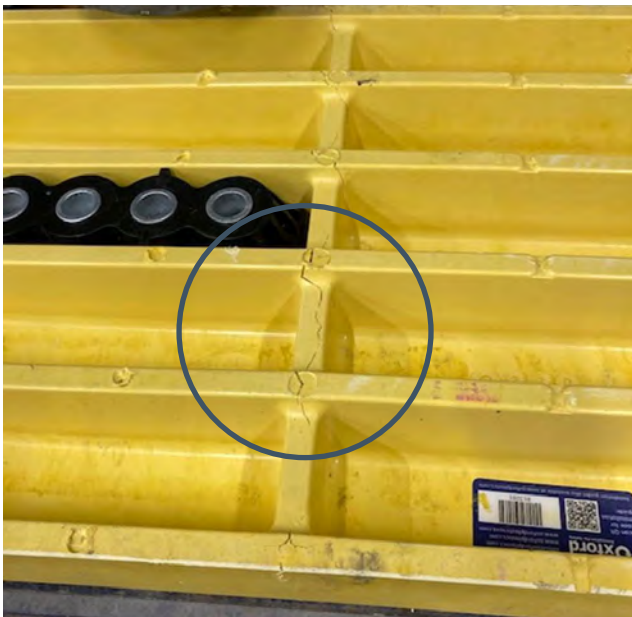
Crack along rib
